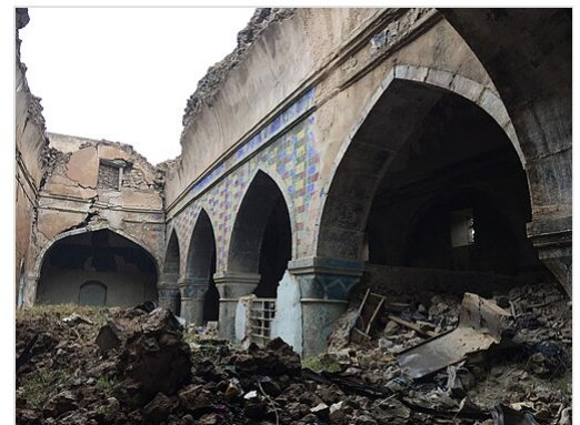
Ruined Sassoon Synagogue in Mosul
